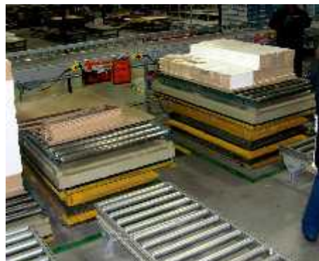
Improvement: Standard powered hydraulic lifts, with conveyor spurs for staging incoming pallets
